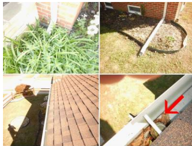
Some Debris in gutter
